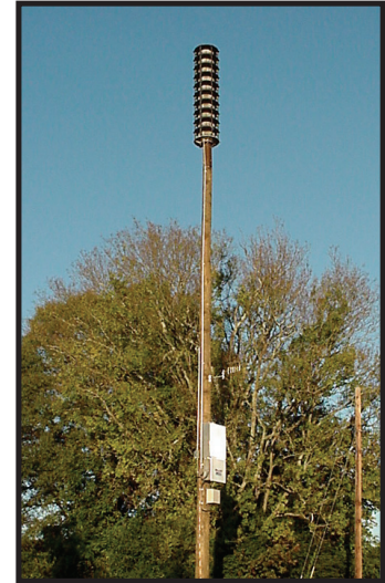
Whelen WPS2910 installed on site in Columbus, Georgia.
